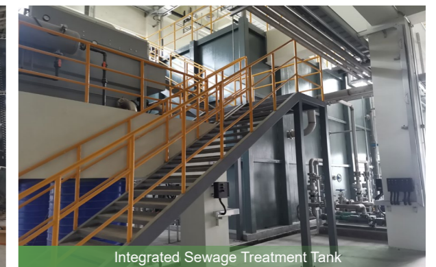
Sewage Treatment Station Conditioning Tank
